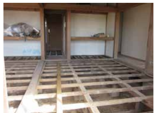
A house whose ground floor was once flooded and yet to be repaired
