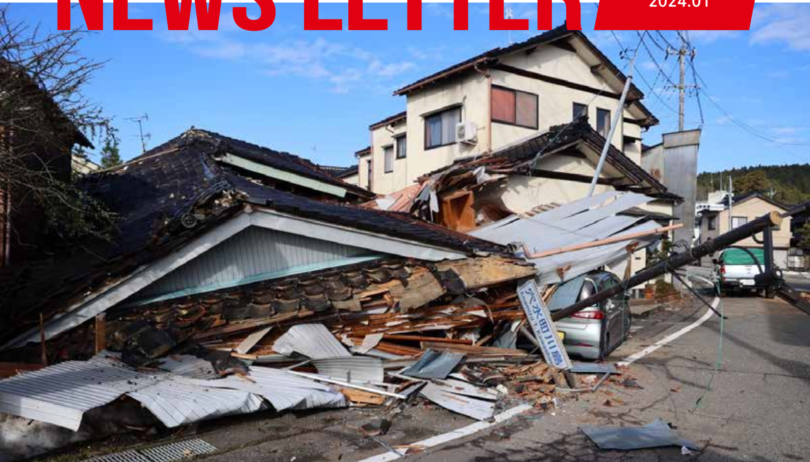
Roads and water access were cut off and houses were collapsed across Noto Peninsula (January 2, 2024)
